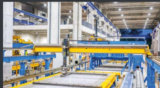
Automated concrete spreader at R3 Precast's facility in Pulau Punggol Barat
